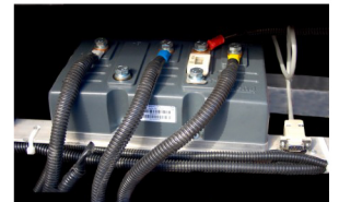
450amp AC Speed Controller
